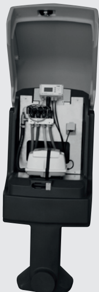
Exterior switch cabinet
